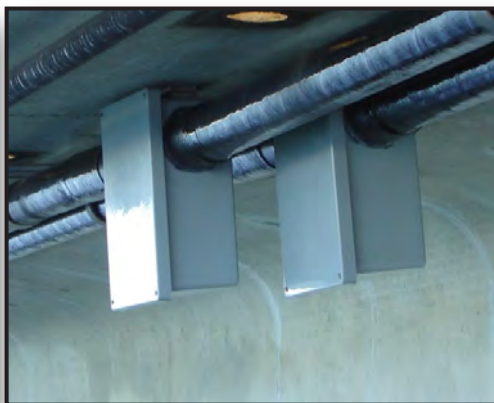
Power Junction Box
