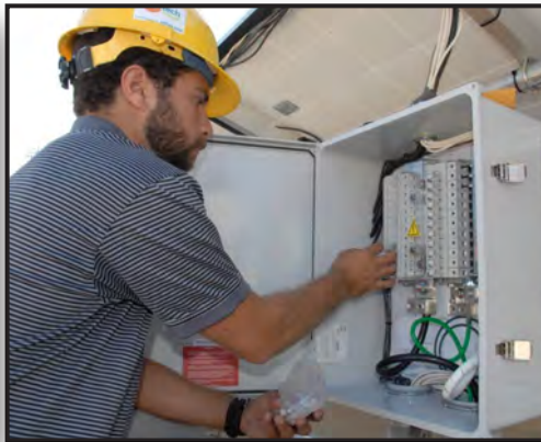
Solar Combiner Box
